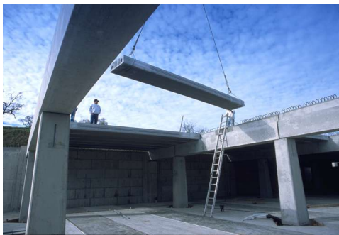
A crane positions a 4-ton plank into the ceiling of the Nickel & Nickel barrel cellar.
